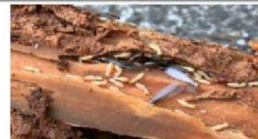
Termites damage houses
