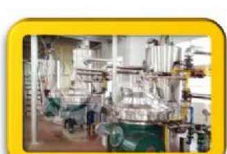
OIL REFINERY INDUSTRY
