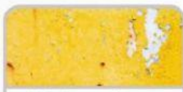
old (chipped) paint
