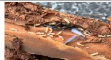
Termites damage houses
