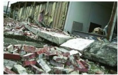
Earthquake damage in Washington in 2001
