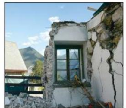
Buildings, bridges, and other structures collapse.
