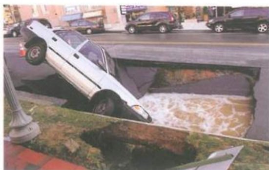
A car falls into a sinkhole
